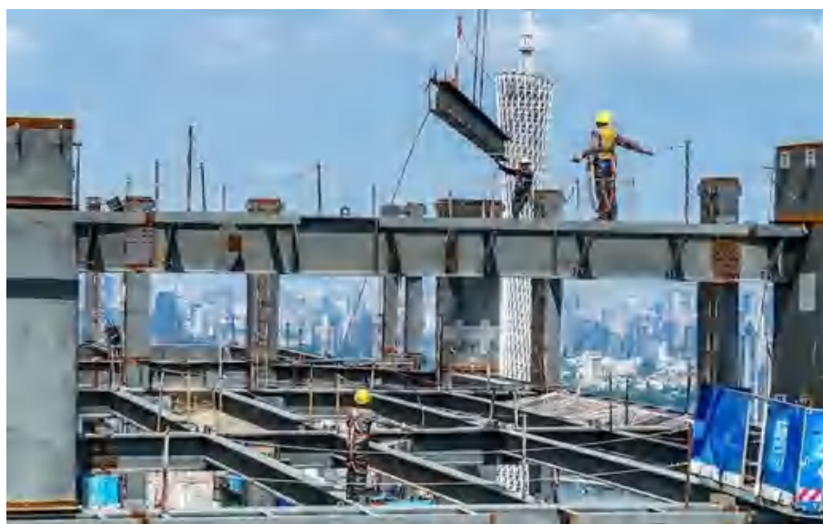
Guangzhou Pazhou Artificial Intelligence and Digital Economy Pilot Zone under construction, Sept. 3rd, 2022. (Source: Visual China Group)
